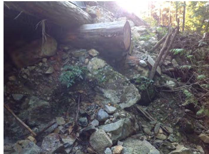
scour under left downstream sill
