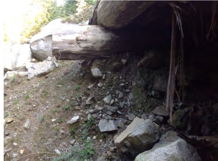
scour under right downstream sill
